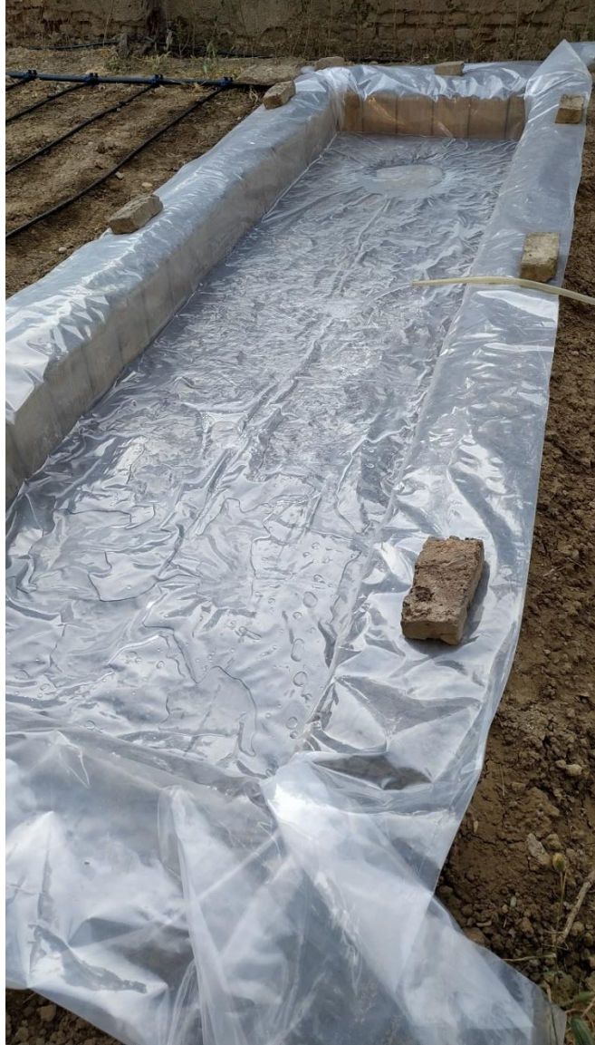
Figure 7: Floating Raft Reservoir and Plastic Sheeting
